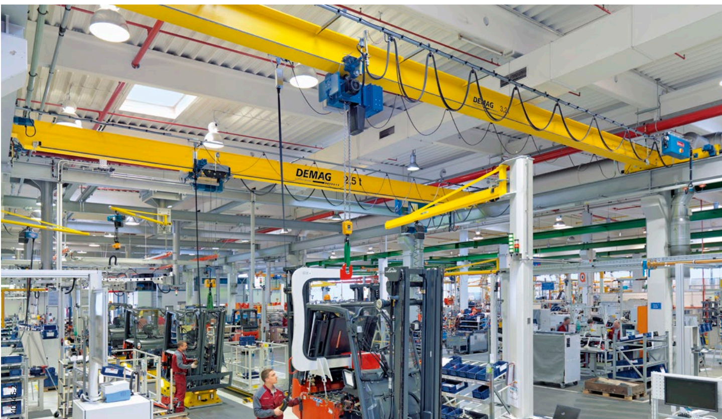
Assembly line for forklift trucks: Crane type EPKE equipped with DC chain hoist
